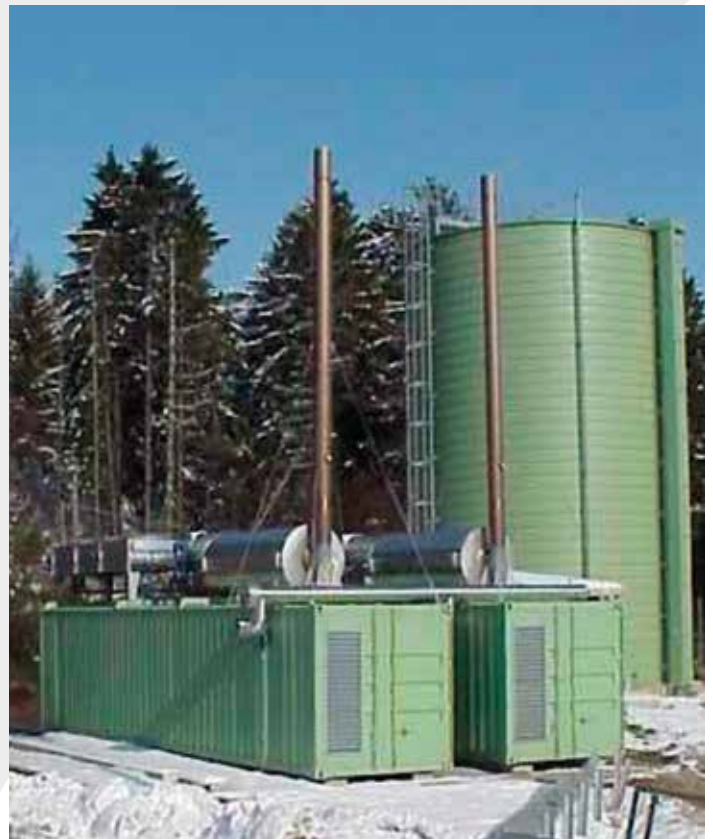
CHP Standard container unit connected to district heating system
